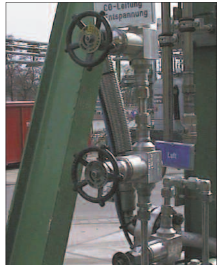
Model 2020 on tanks discharge - High pressure (225 bar) carbon monoxide isolation - Germany
