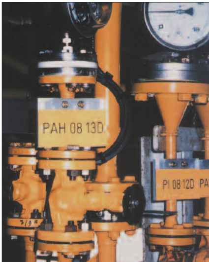
Pressure transmitter valve isolation on gaseous chlorine - France
